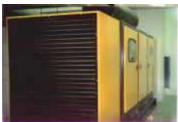
GE 800 Kva City Bank Moscou
